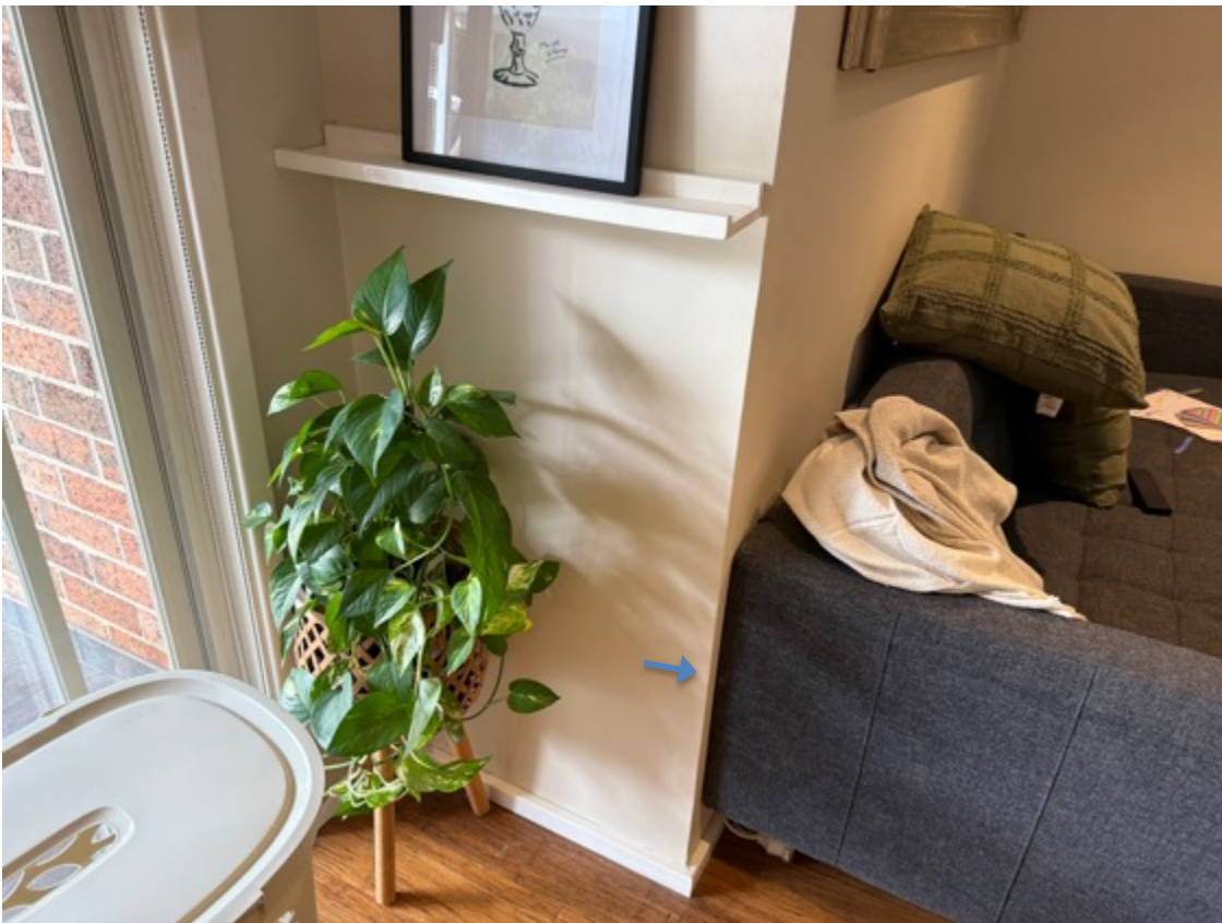
Internal surfaces display low level paint blemishes, consistent with age.
