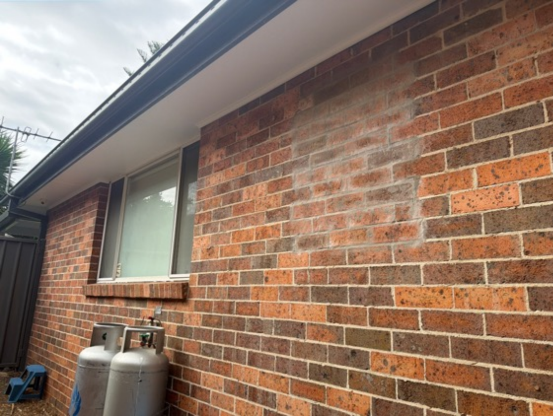
Left side elevation mid-sections n brickwork has been patched here.
