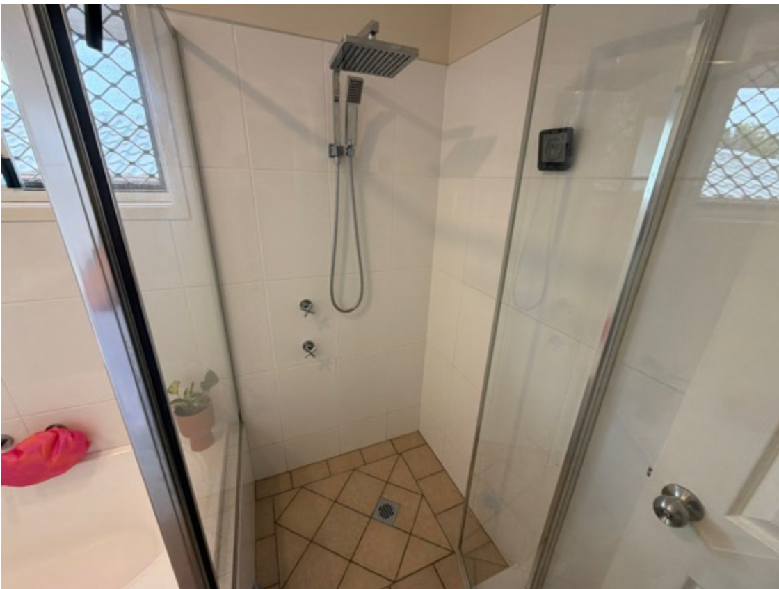
Hot and cold water services tested, functioned at the time of inspection.
