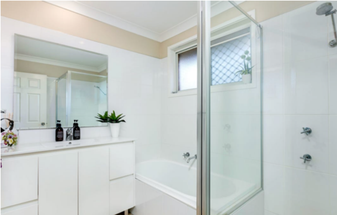
The common bathroom area tested for leaks, fixings and stability was issue free at the time of inspection.
