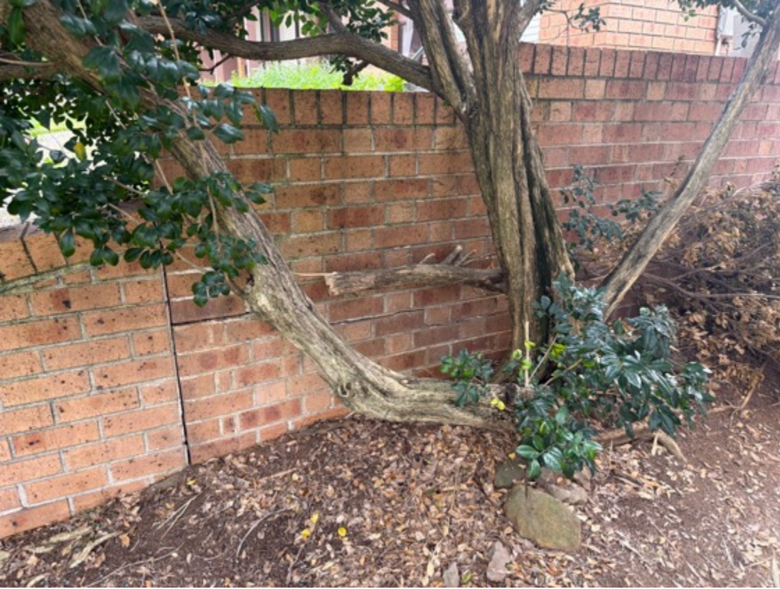
The front left side retaining wall has cracking visible - requires remedial works.
