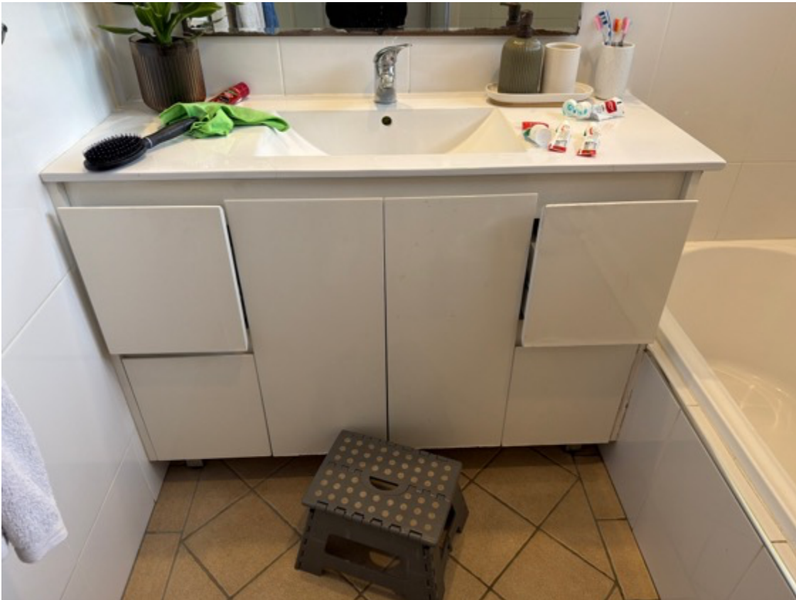
Water pressure tested, is sufficient.
