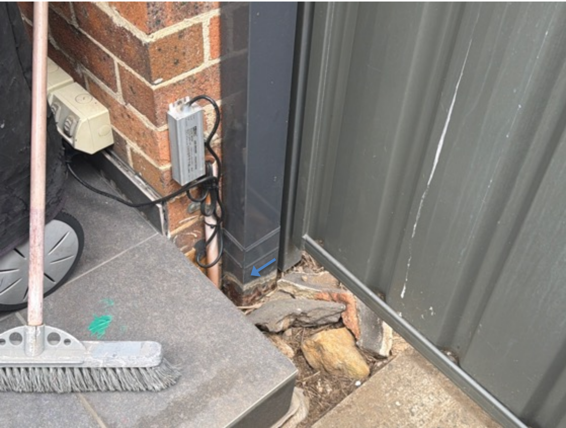
The rear left side downpipe has surface rust visible at the base.
