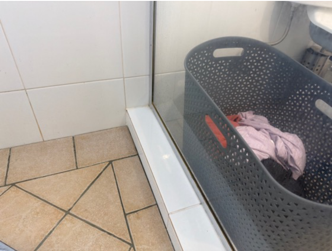
Isolated sections of tiles are chipped, consistent with age, example shower hob above.
