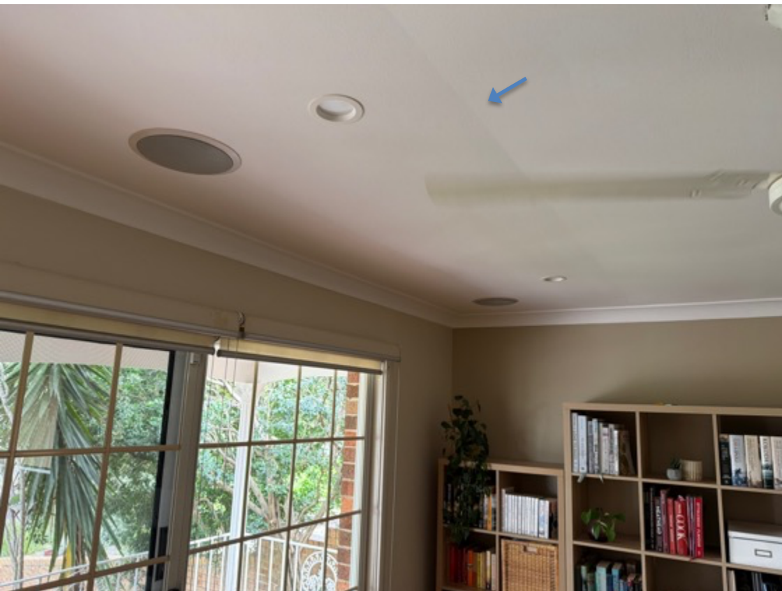
Internal plasterboard and cornices display minor imperfections.
