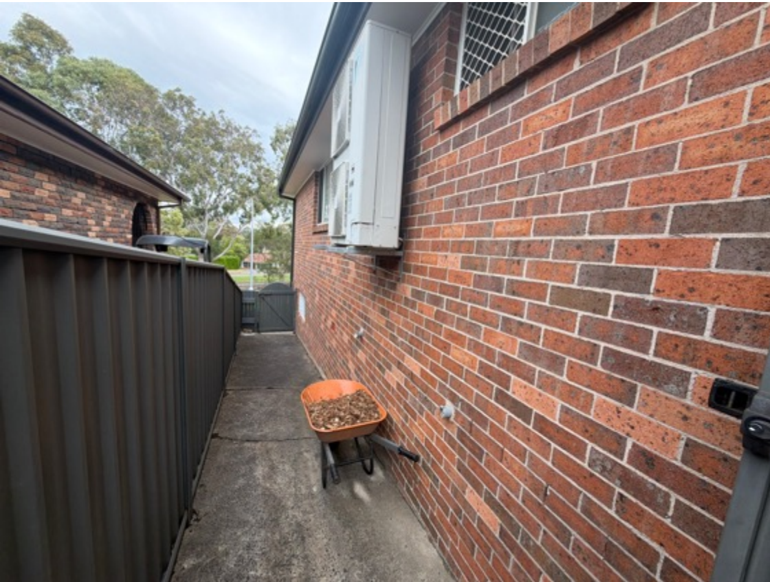
Site fences are in serviceable condition, isolated sections have a slight inward lean, consistent with age.
