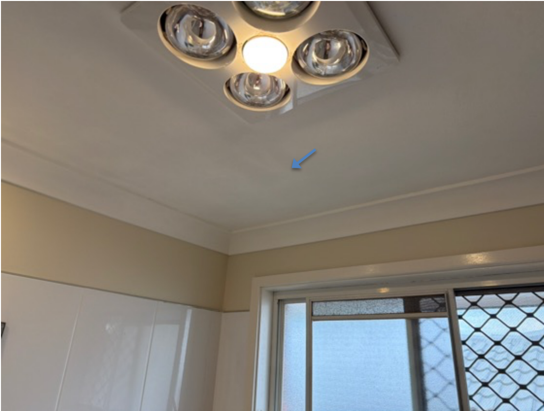
The ceiling paint is patchy.
