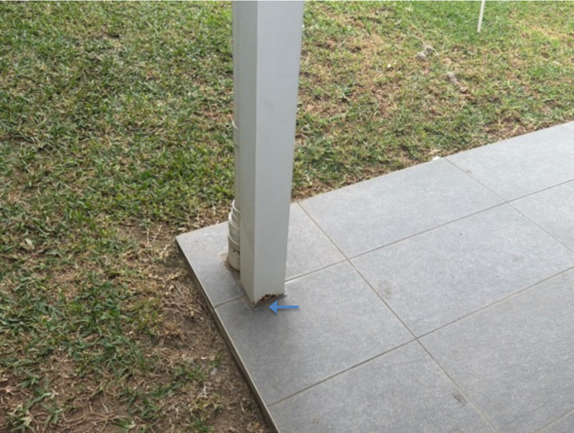
Base of pergola posts have low level surface rust visible.
