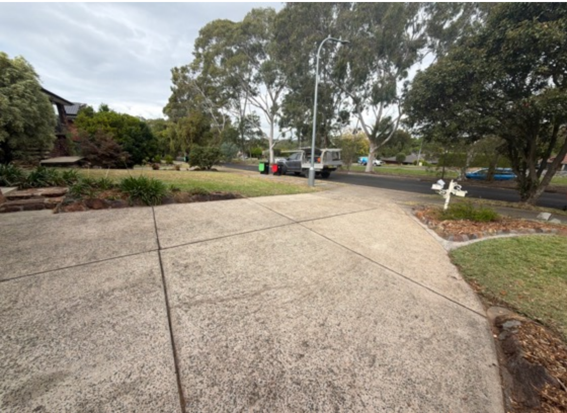
Exterior concrete presents in satisfactory condition for the age - isolated sections are cracked and undulating (consistent with age.)
