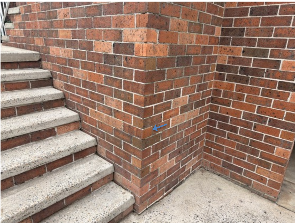
Isolated sections of external brickwork displays category one cracking (front elevation example above.)
